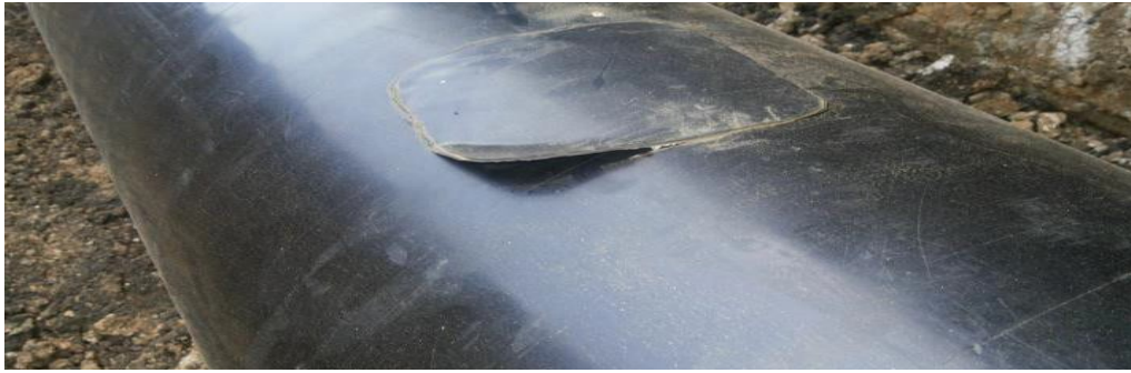
Figure Adhesive failure
